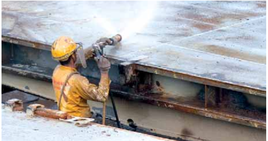
Hydro-blasting is employed for projects whenever feasible to prevent grit and dust dispersion.
