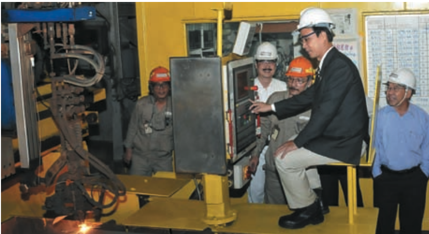
Nguyen Quynh Lam, CEO of Bien Dong Production & Operating Company, activates the cutting of the first steel for the KFELS SSDT™
