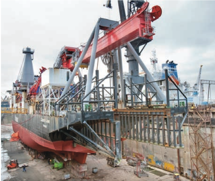
The repair and modification works on trenching support vessel, Calamity Jane, were completed without incidents
