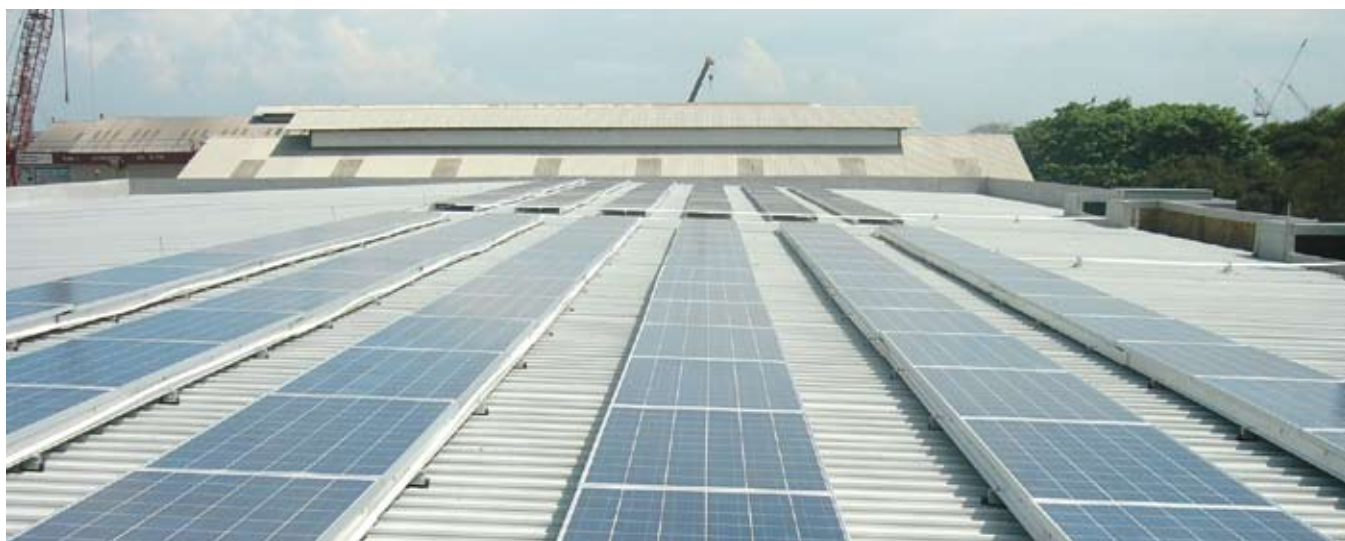
At KOMtech, two photovoltaic (PV) power plants were installed on its rooftop to convert solar power into electricity
